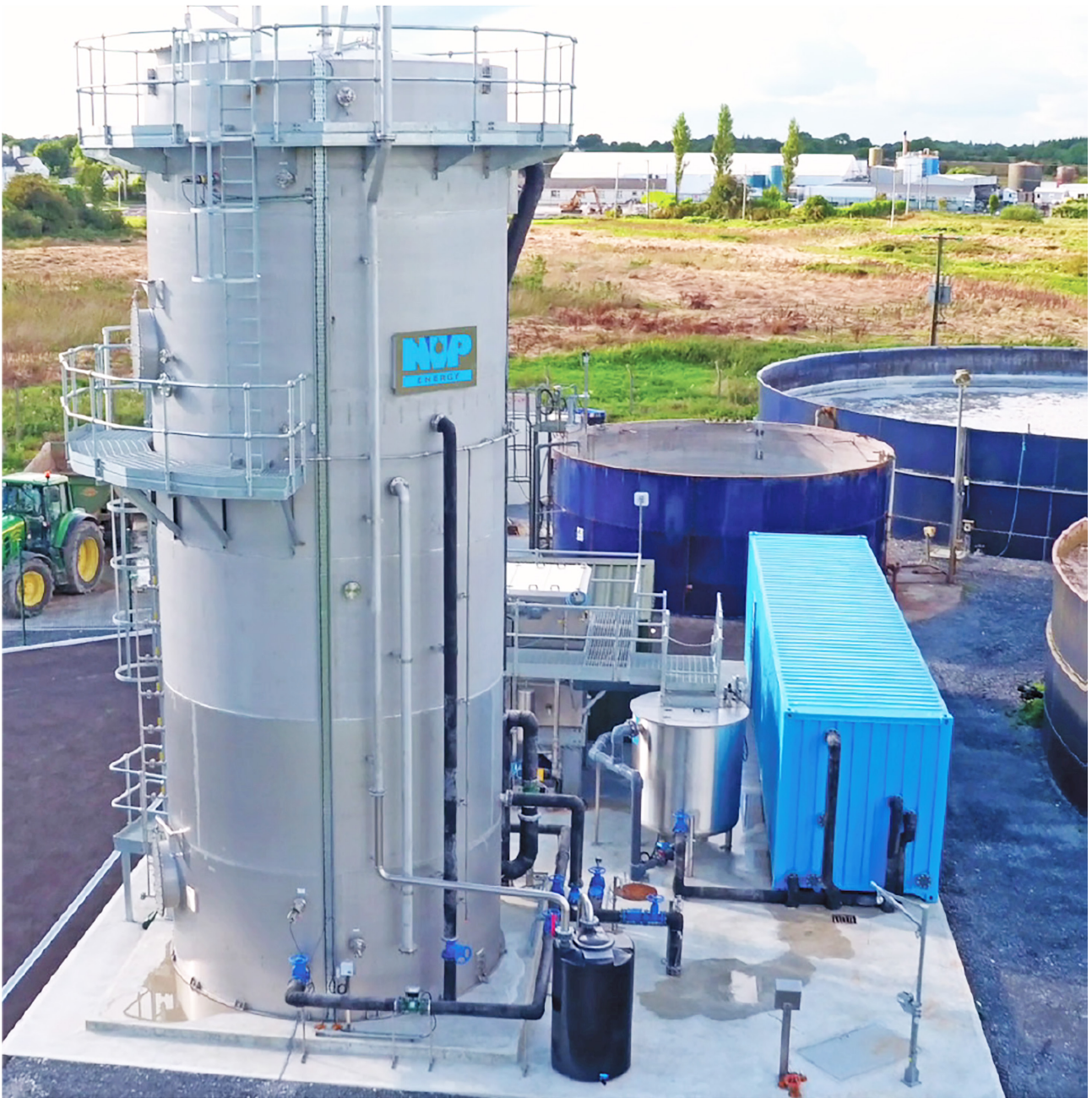
NVP Energy module and container
