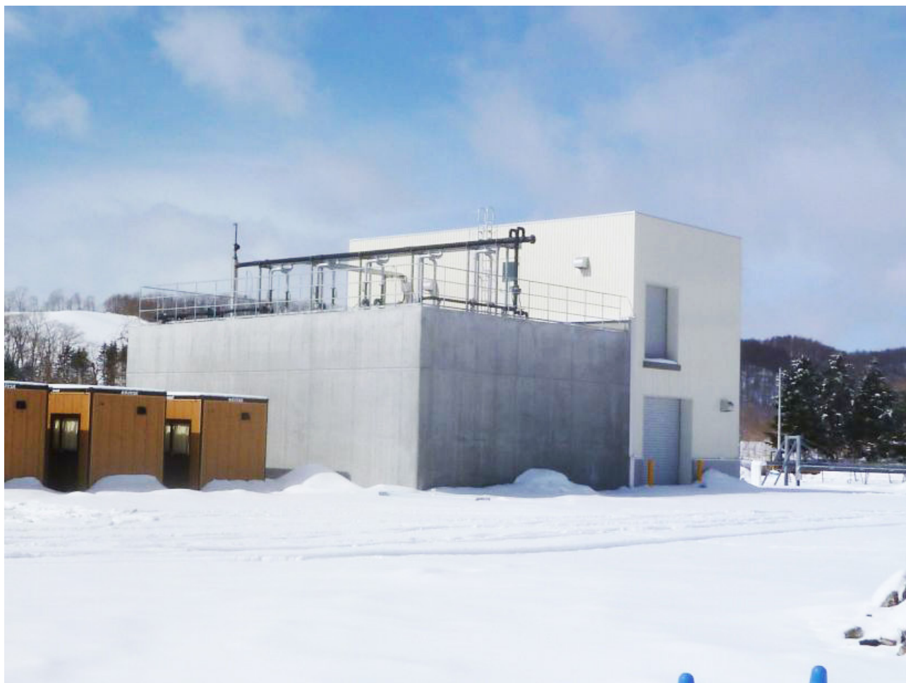
New membrane tank
